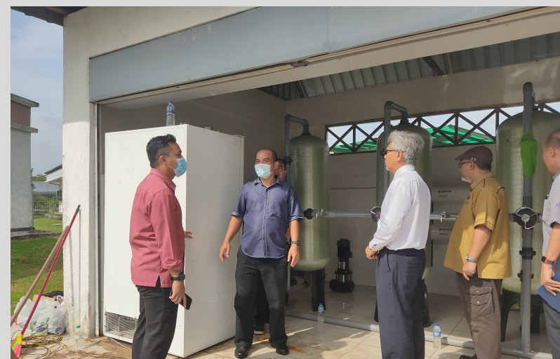
SESI LAWATAN TAPAK PROJEK BAGI GERAN KONTRAK UTHM (GROUNDWATER SUPPLY AND TREATMENT SYSTEM DEVELOPMENT FOR MASJID SULTAN IBRAHIM UTHM) TARIKH : 06 OGOS 2020 (KHAMIS) TEMPAT : MASJID SULTAN IBRAHIM, UTHM
